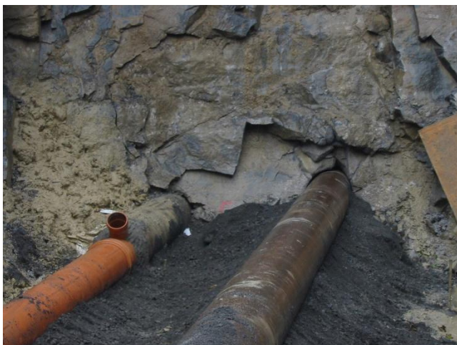
N7 crossing in Galway for commercial development for sewer and surface water connections completed
